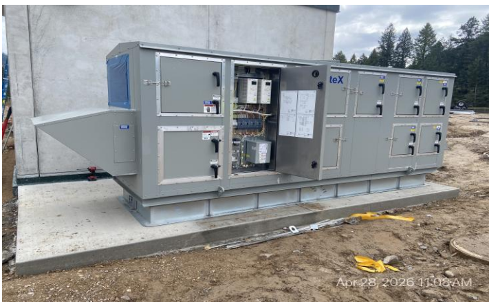
Air Handler for Headworks Building
